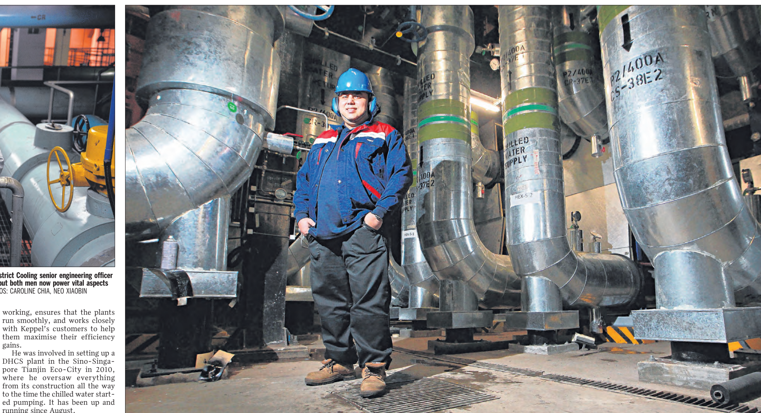
efficient chiller equipment planned for next year. Keppel, which is looking into new sites for DHCS facilities,
