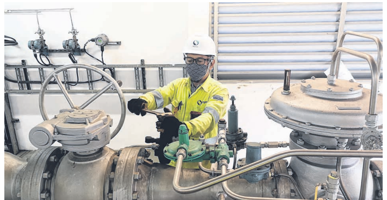
A member of the SP Group gas operations team at an offtake station conducting checks on the gas regulators. The utilities firm is adjusting the gas pressures within the transmission and distribution network for residential and industrial customers as Singapore enters phase two of its reopening. PHOTO: SP GROUP
