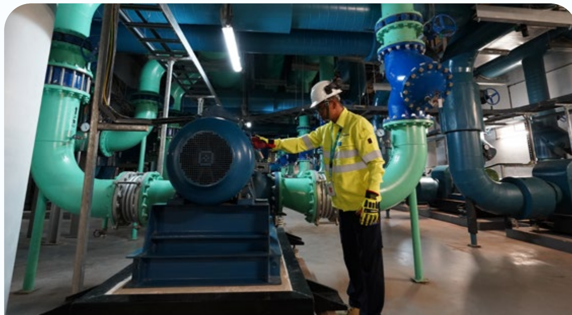
The distributed district cooling system at Tampines Central
