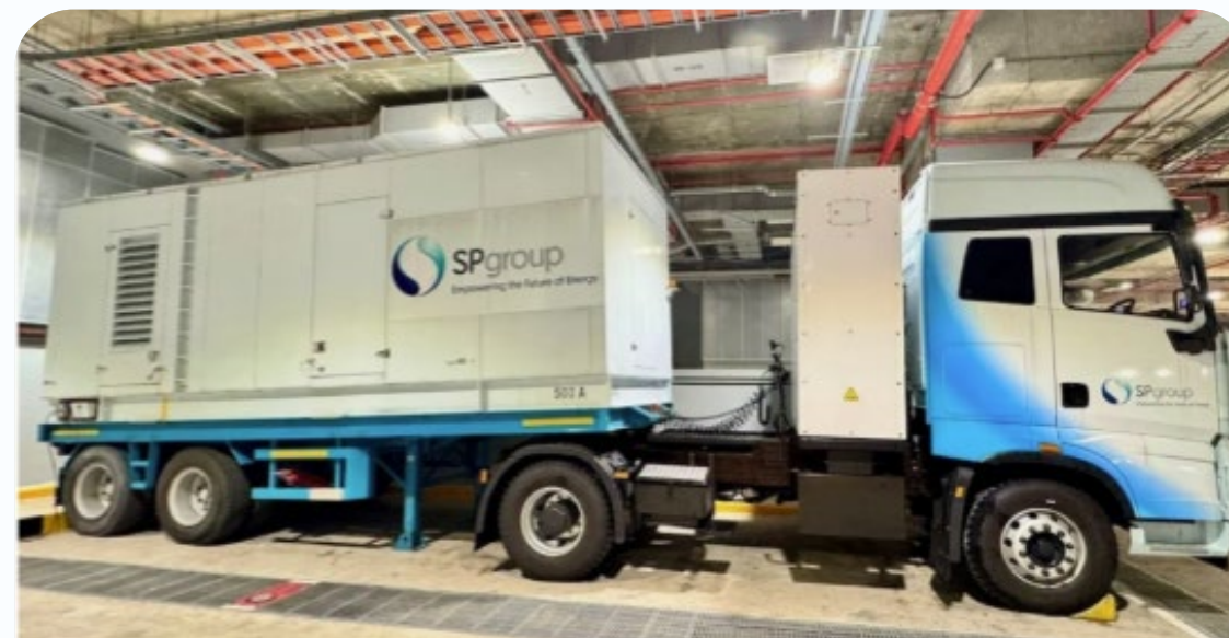
SP Group deploys e-PM to transport generators during supply restoration. The e-PM is fitted with advanced safety features for enhanced stability.
