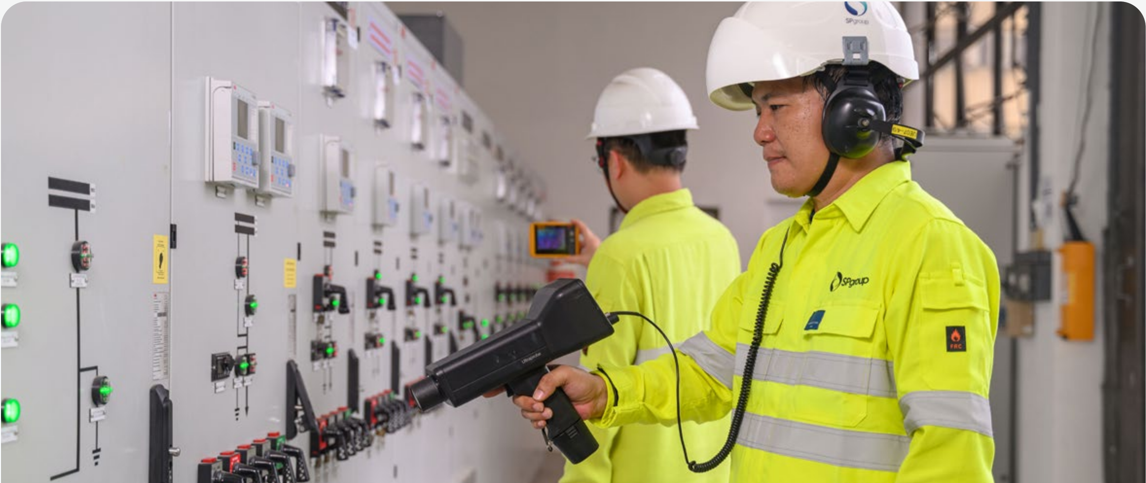
Before adopting new technologies, Eric Lee (front) and his colleagues previously used portable diagnostics tools to detect anomalies in the electrical equipment in substations
