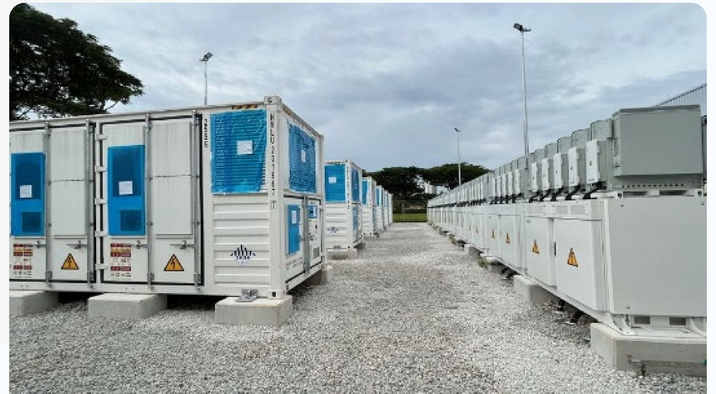
Battery energy storage system at Kallang, supporting grid resilience
