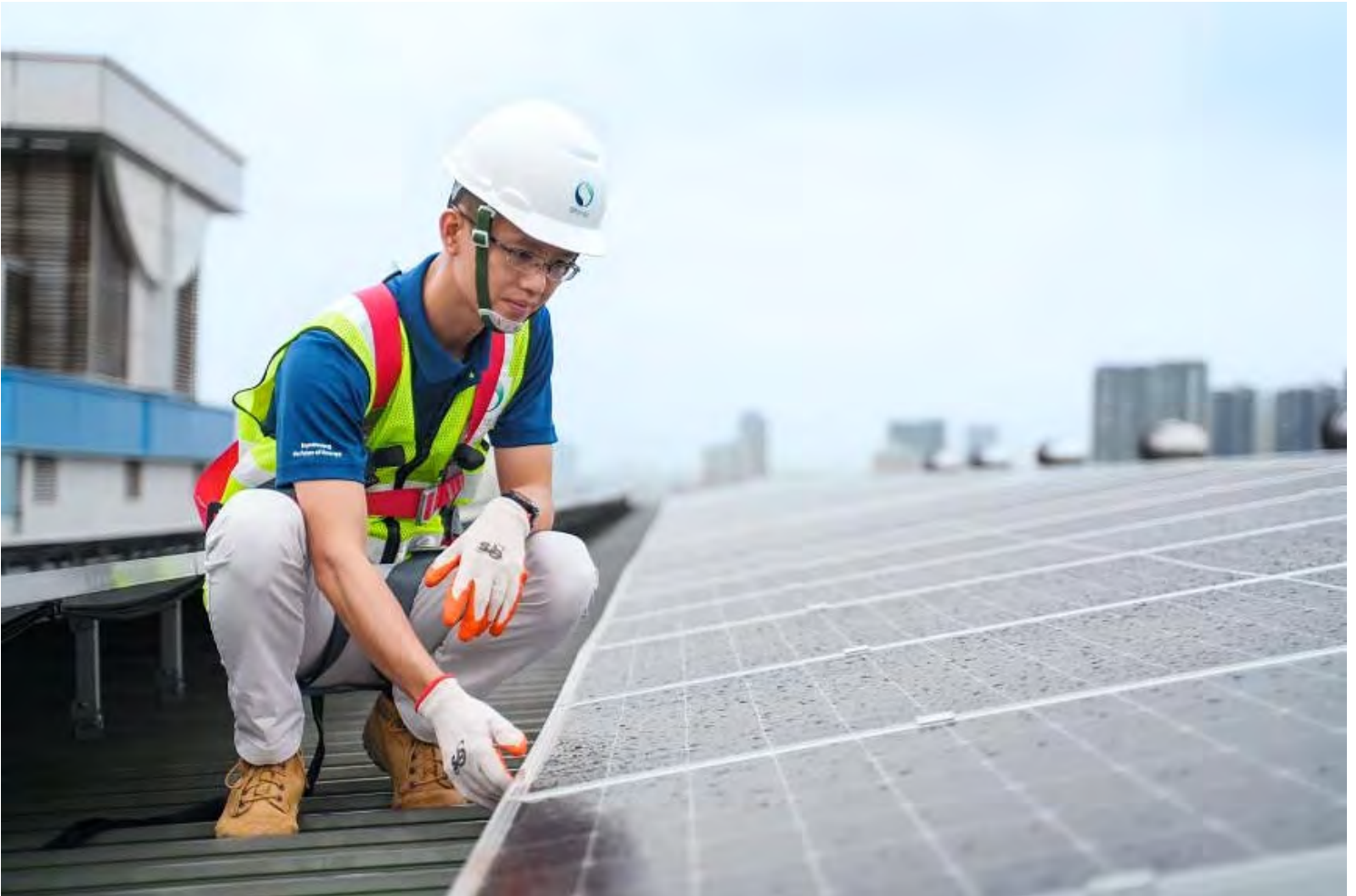
Part of principal engineer Xcel Lai's job is to identify and optimise underutilised spaces so that solar panels can be deployed to generate renewable energy. PHOTO: SP GROUP
