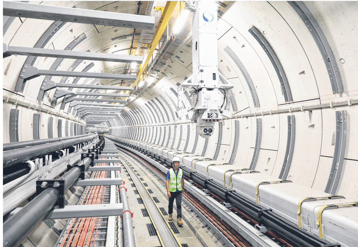
SP Group's underground transmission cable tunnel system that brings electricity to consumers. The power grid operator is looking to build transmission lines to neighbouring countries and using renewable energy credits for power trading to obtain green power for Singapore's use. ST PHOTO: ONG WEE JIN
