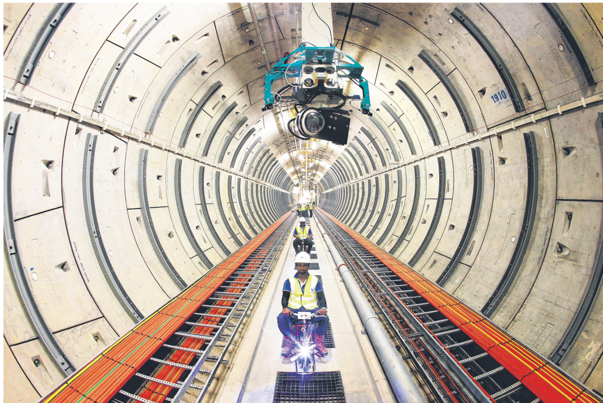
SP Group staff riding electric bicycles yesterday in the tunnel network of the Underground Transmission Cable Tunnel Project. Above them is a prototype model of an automatic inspection vehicle, the final version of which will be used to monitor the tunnels for water seepage and fires. PHOTO: LIANHE ZAOBAO
