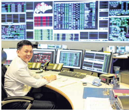
Energy Market Authority control manager Derrick Lim in a room that oversees the transmission of high-voltage power. PHOTO: ENERGY MARKET AUTHORITY
