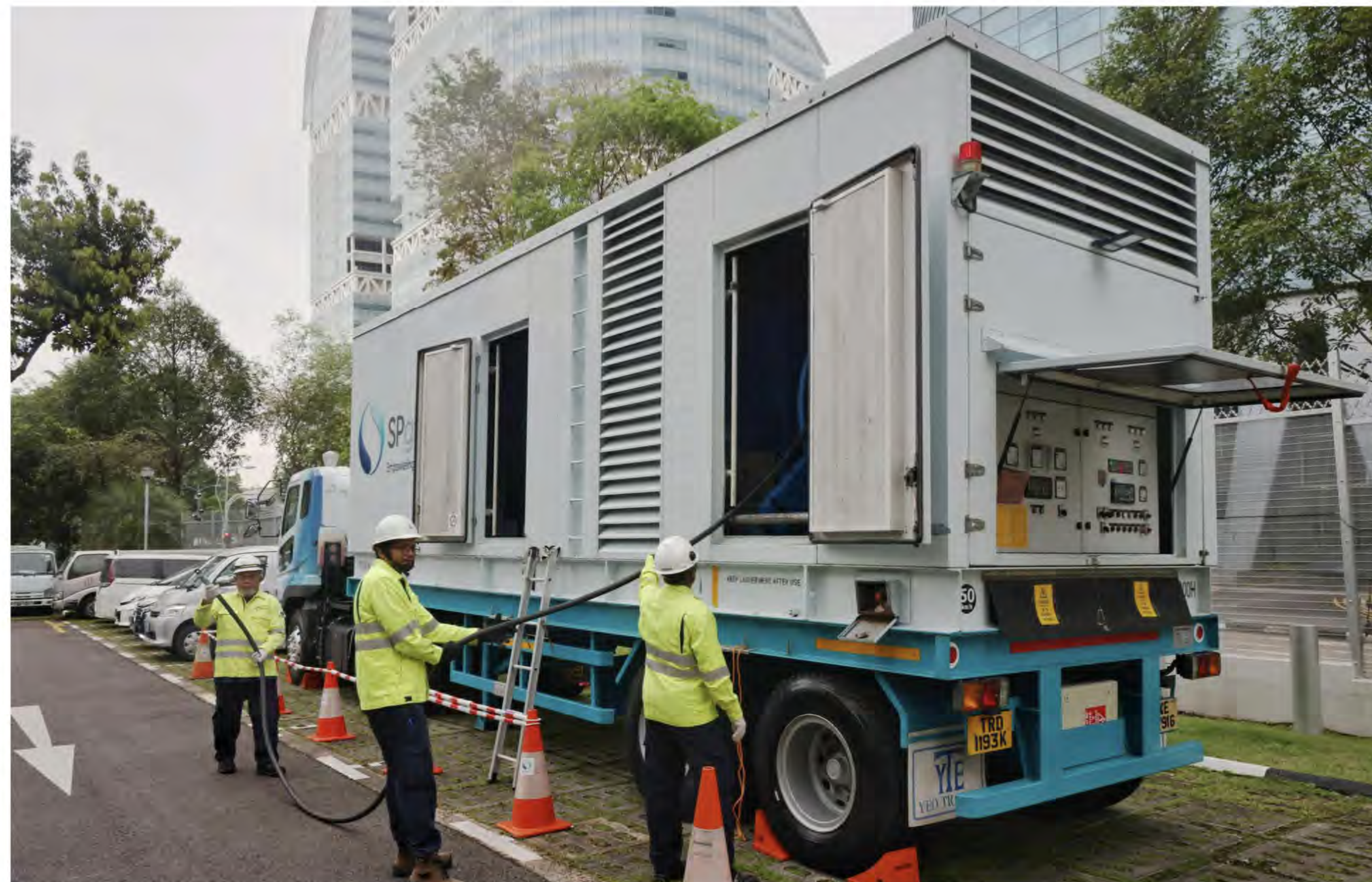
SP Group staff demonstrating how they set up a mobile power generator on Jan 24. This year's Total Defence drill – Exercise SG Ready 2025 – is aimed at encouraging all to plan for potential disruptions, strengthen business continuity plans for power disruptions or phishing attacks, and prepare to respond effectively. It will run from Feb 15 to 28. ST PHOTO: JASON QUAH
