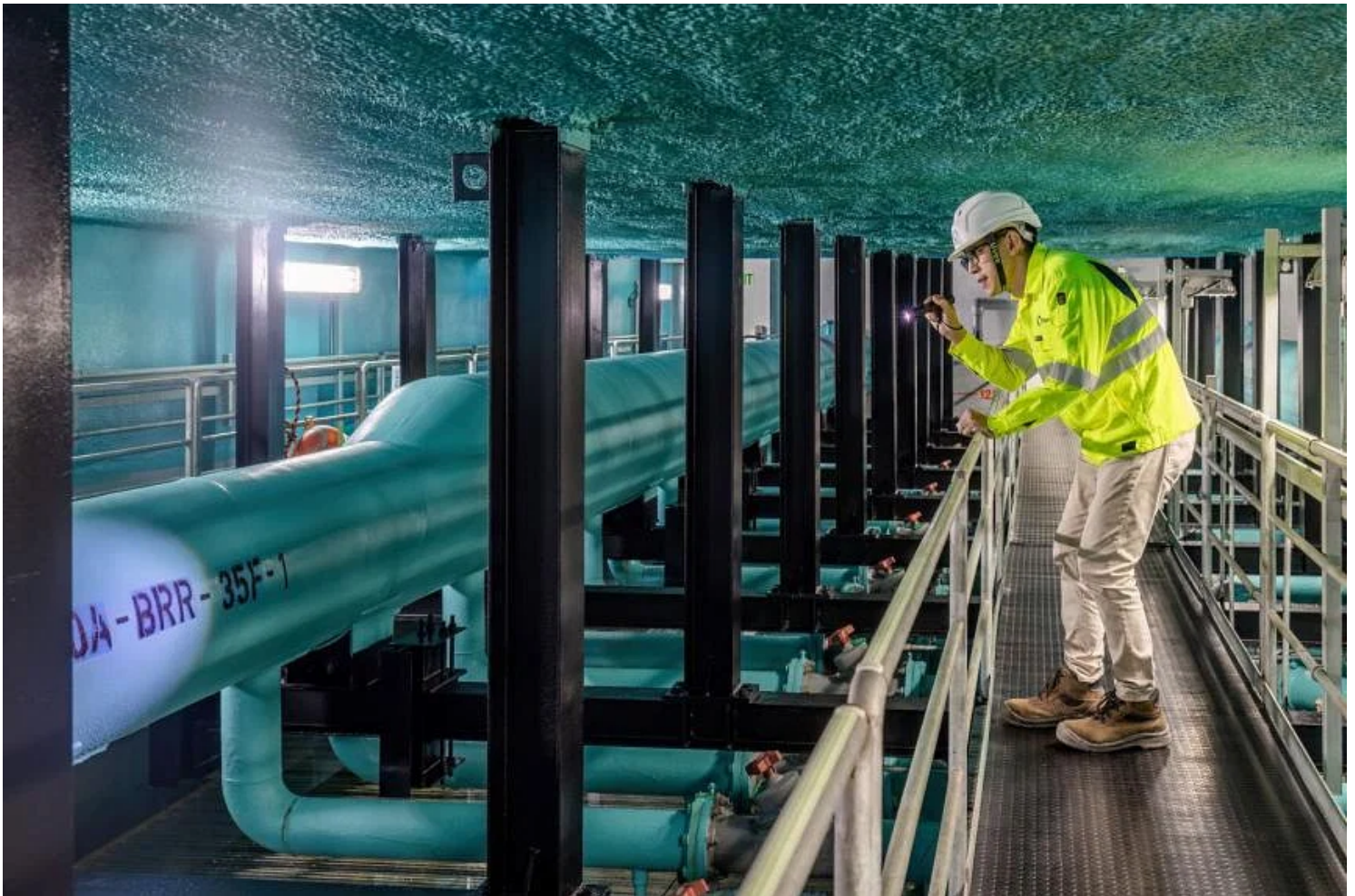
Mr Liu Yue inside one of the thermal storage tanks in the world's largest underground district cooling network operated by SP Group PHOTO: SP GROUP
